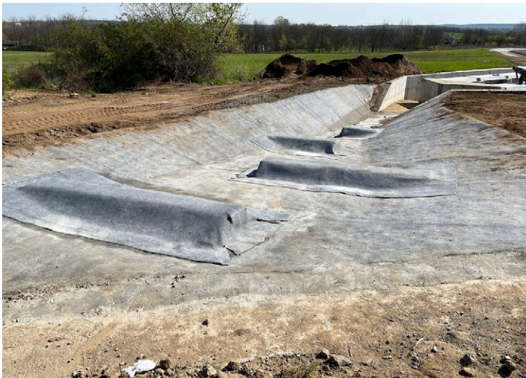
Baffles covered in CCX-M™
